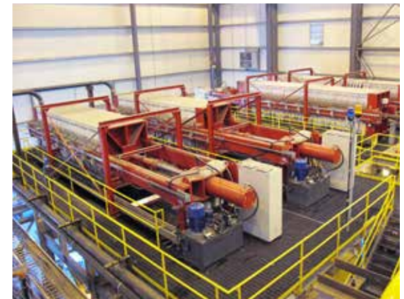
Utah filtration plant
