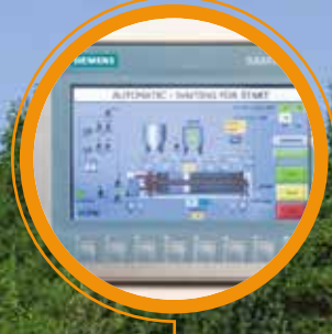
ALLEN BRADLEY AND SIEMENS TECHNOLOGY FOR PLC
